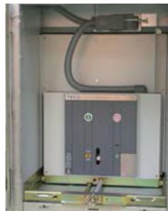
Circuit breaker compartments
