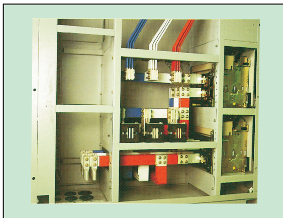
ACB Zone、Busbar Zone and Cable Zone
