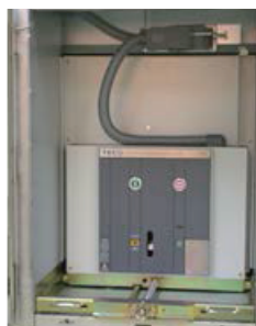
Circuit breaker compartments
